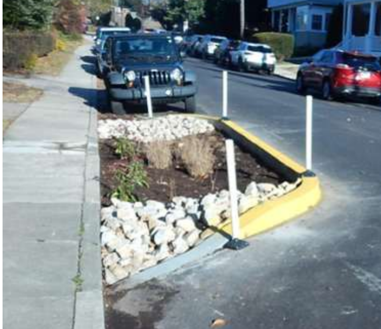
Grayling Ave, Narberth—rain garden bumpouts, stormwater management project funded through a 2025 LVR grant
