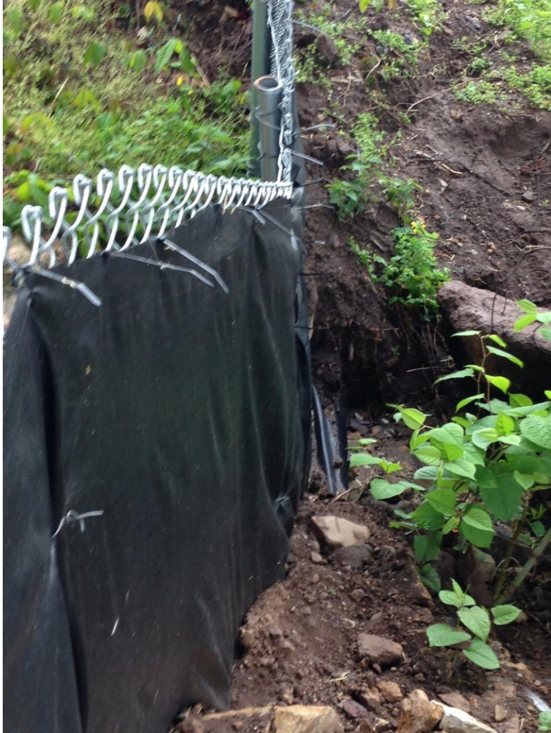
Super Silt fence that has been undermined.
