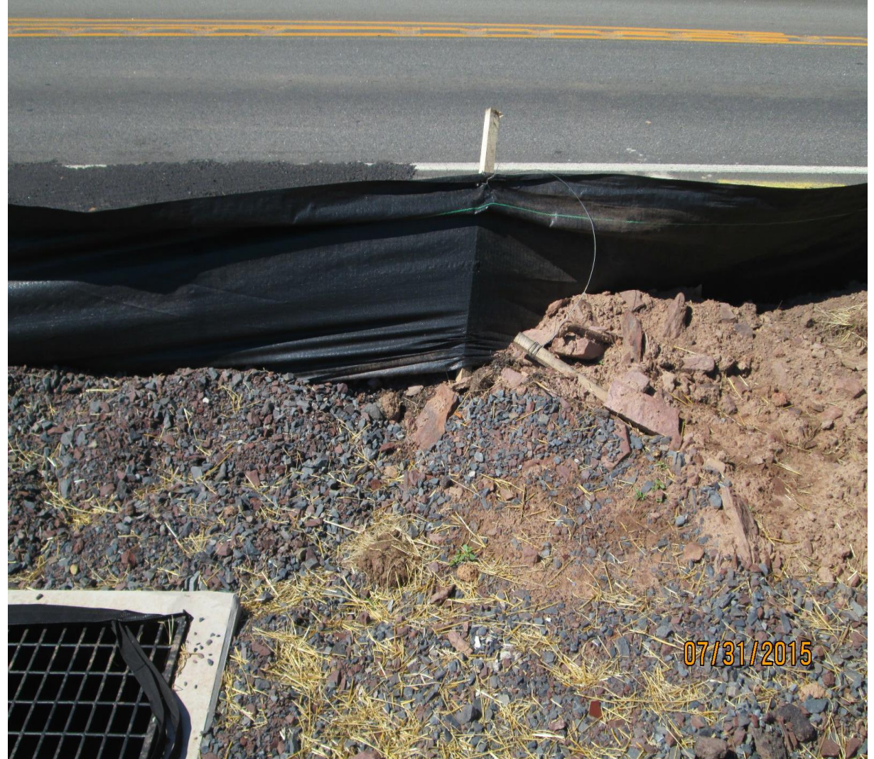
Reinforced silt fence that isn't entrenched and stakes have been pulled out.
