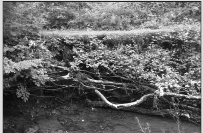
Perkiomen Creek pre-construction: bank erosion baring tree roots at the stream's bend, where a log vane deflector and root wads were later installed.
